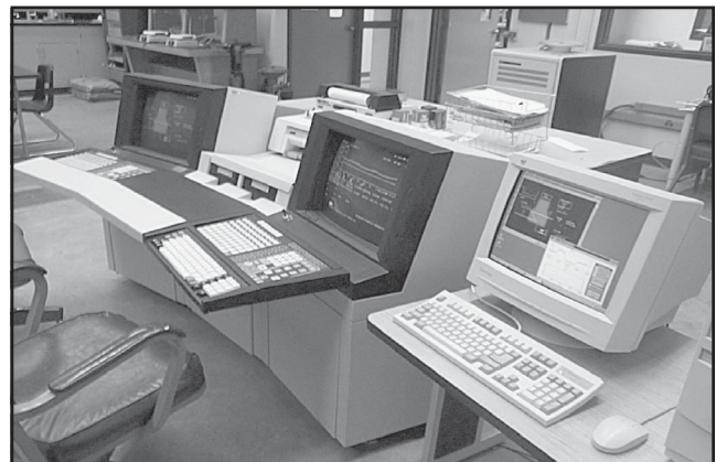
Figure 2. Representative cluster of Universal and Global User Stations for ASU's TotalPlant Solution System.
